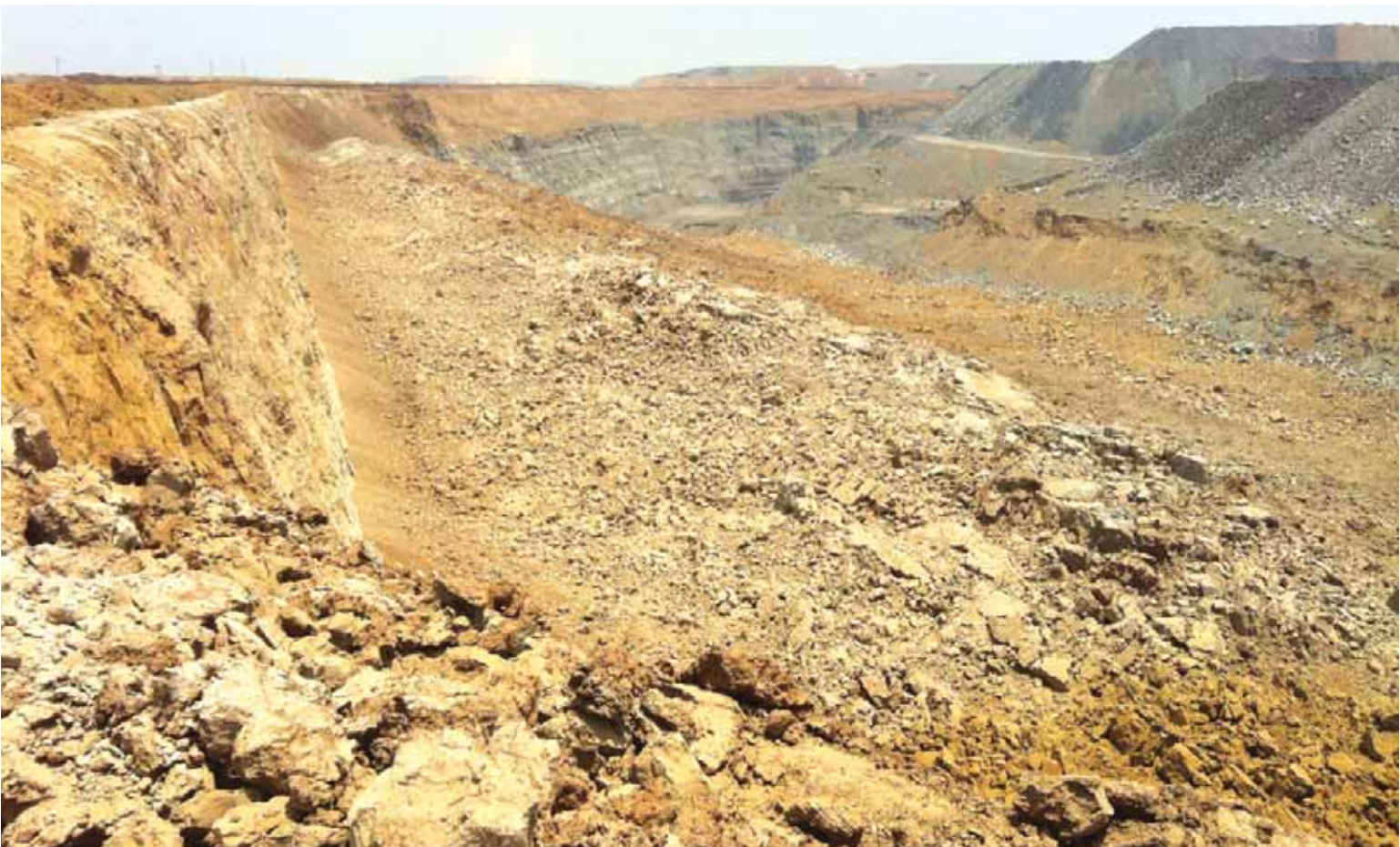
One of the most useful applications for electronic systems is in large-tonnage blasting where electronics can deliver cost efficiencies by reducing delay scatter, which will improve fragmentation and ultimately reduce the amount of bulk explosives required.
